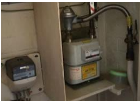
Asbestos panelling around a gas meter
