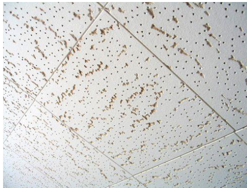
Asbestos containing ceiling tiles
